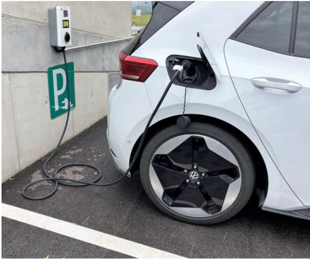
Expansion of charging infrastructure © PORR
