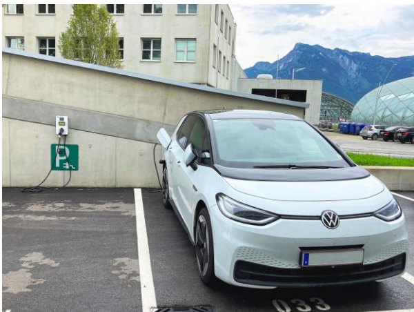
PORR charging points in Salzburg © PORR
